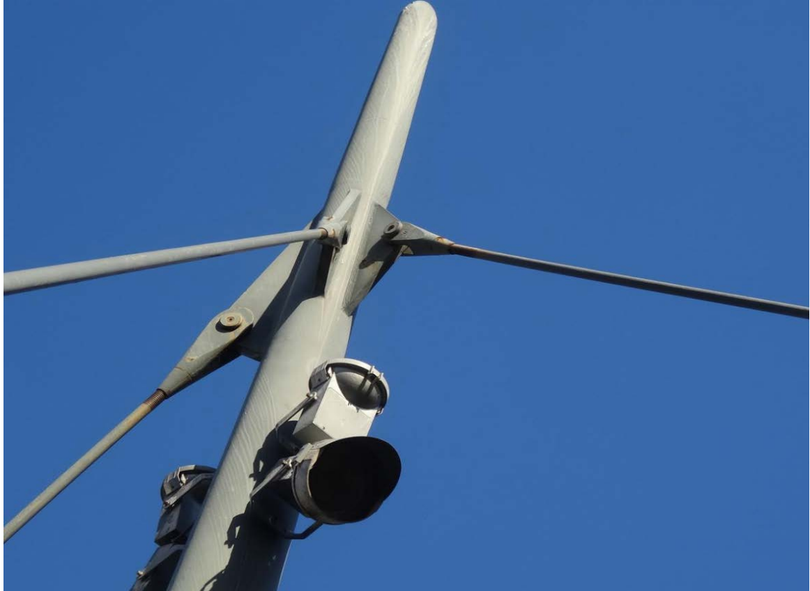
Mast and steel support tendons to be cleaned and repainted
