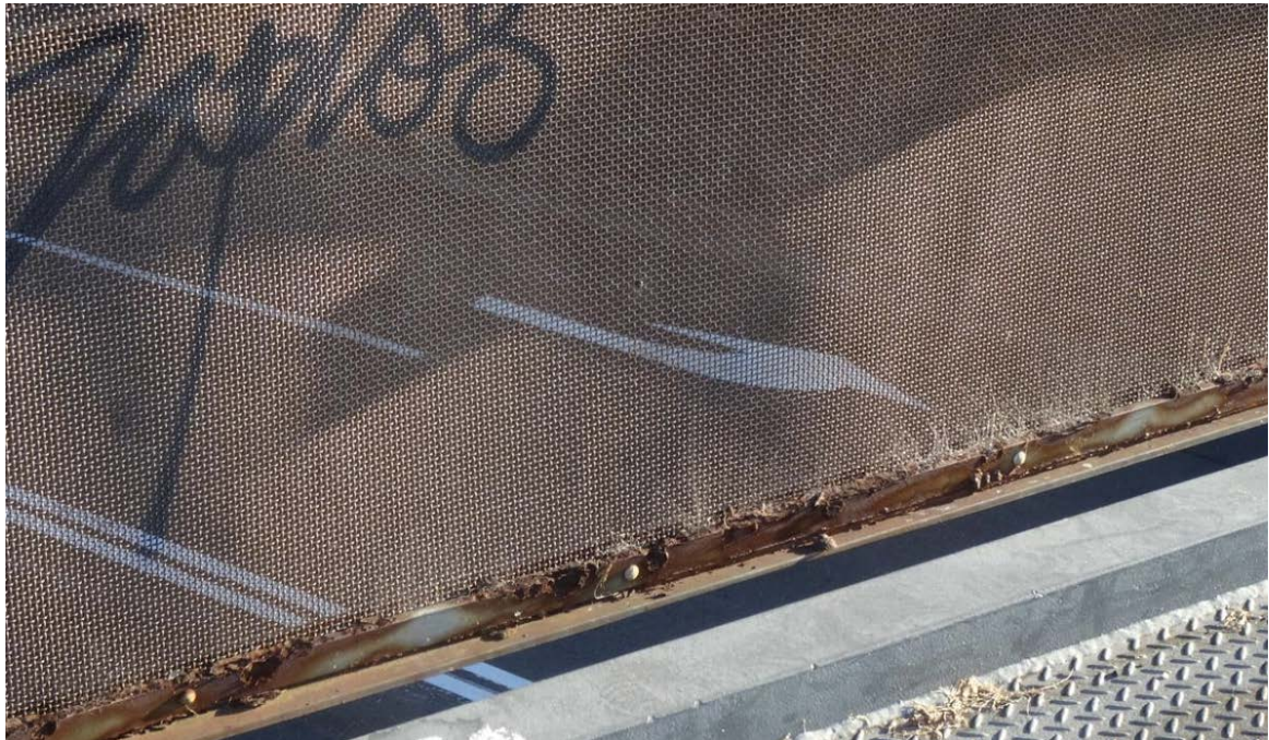
Fence support angles to be replaced
