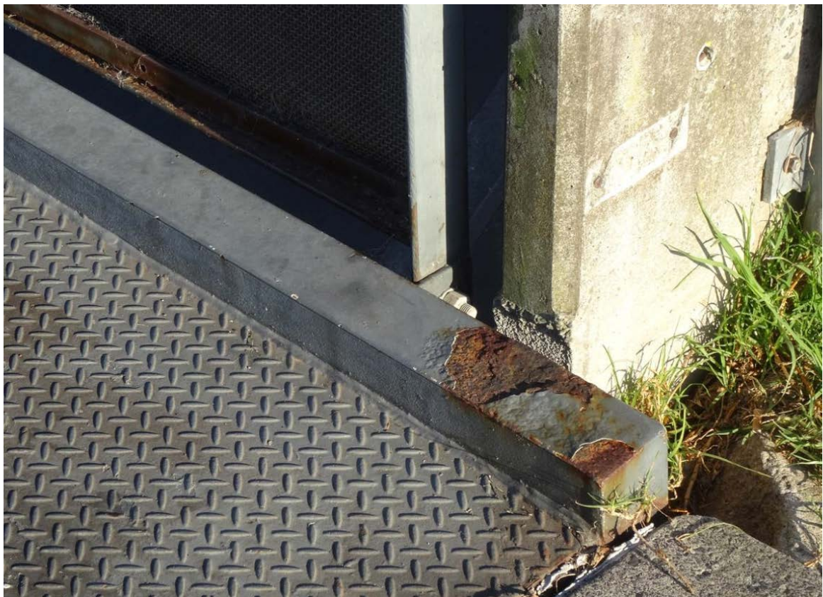
Concrete abutment and lawn to be rebuilt
