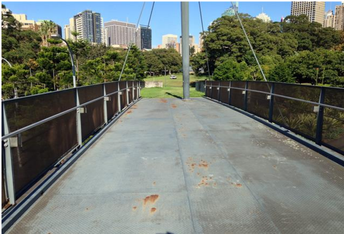
Bridge deck with areas of rust to be treated and deck repainted
