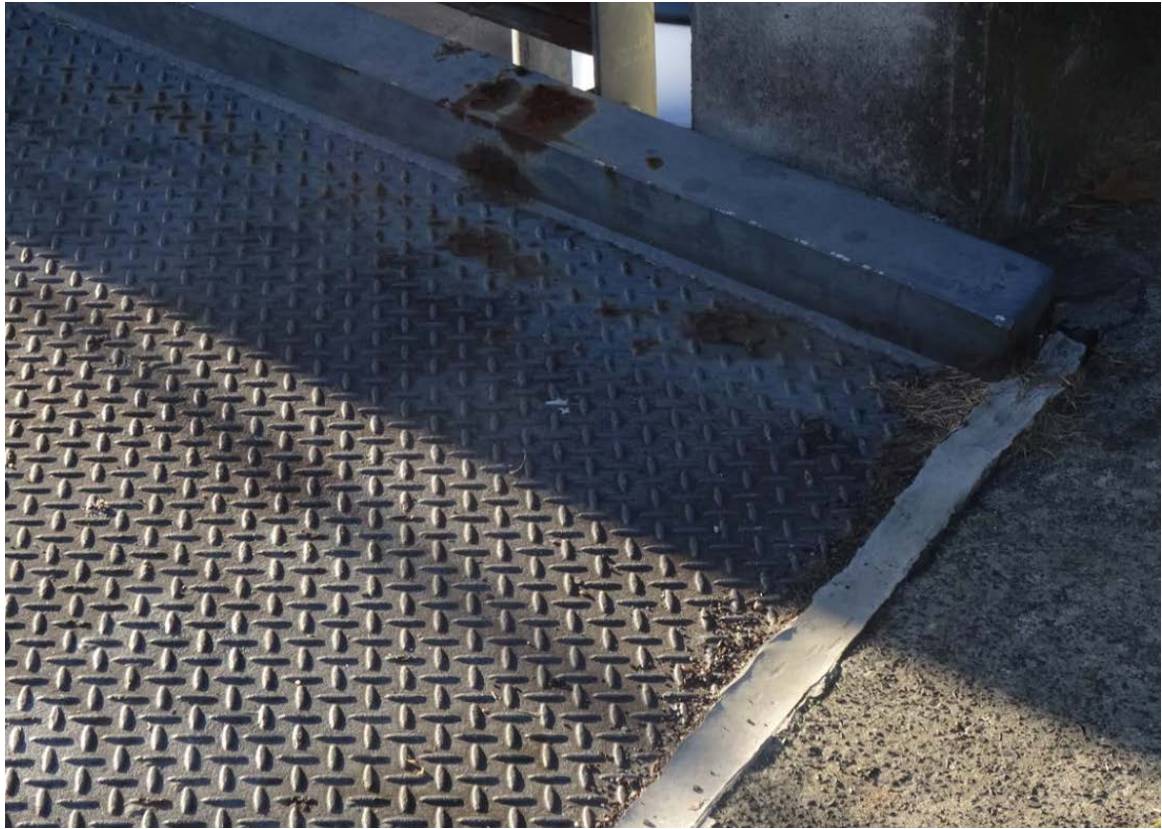
Bridge joint sealant to be removed and replaced
